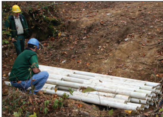
Figure 8.8. PVC pipe bundle installed in ephemeral channel, folded over itself to ensure channel bed is covered and top pipe layer is flat across the top.
