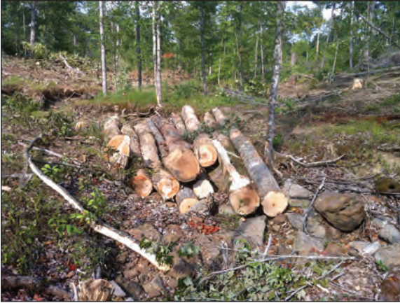
Poles temporarily set in place with a forwarder to cross a small ephemeral channel.
