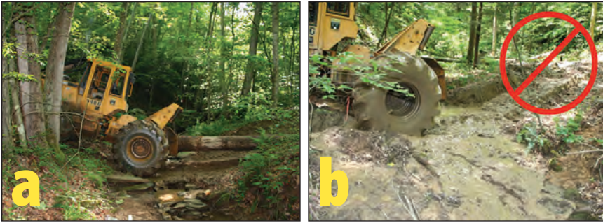
Figure 8.19. Stream with natural rock bed used as a skidder crossing (a). Fords with soft beds are not allowed and poles or other materials must be used to provide proper flotation on stream or channel beds (b).
