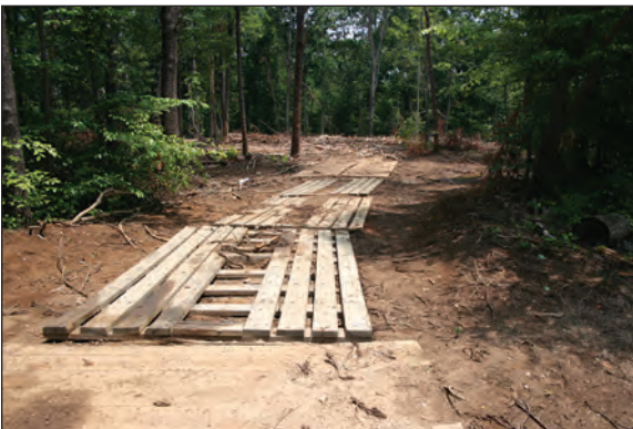
Wood panels used along a haul road to provide flotation for trucks moving from a public highway to a landing.
