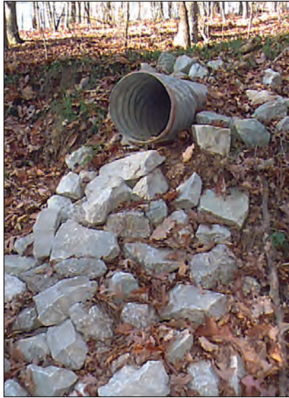
Figure 9.14. Rock used to reduce gully erosion from forming directly below a culvert outlet.
