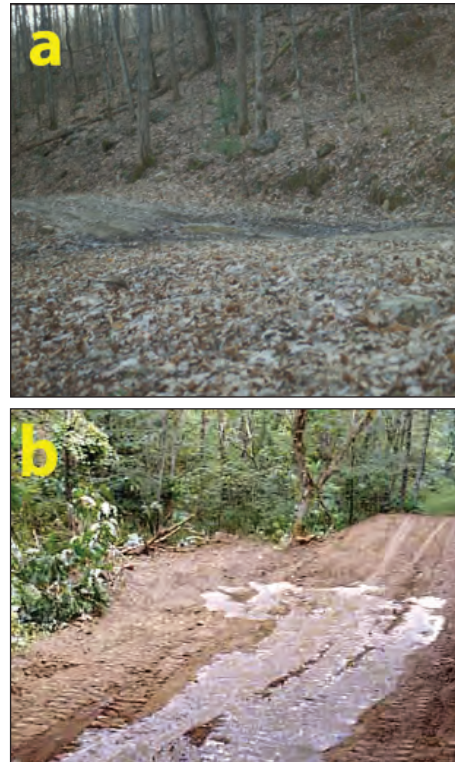
Figure 9.9. Older broad-based dip constructed on an unimproved haul road (a), newly formed broad-based dip showing runoff moving across angled dip (b).
