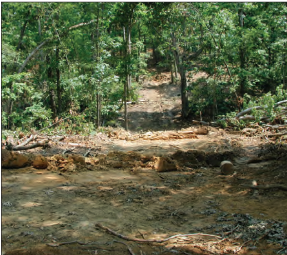
Figure 9.19. Temporary water control structures on a skid trail that will be in place for two weeks before final retirement work will be implemented.
