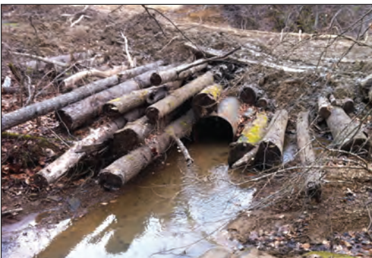
Figure 8.13. Poles used to fill around pipe avoiding depositing soil into stream or channel.
