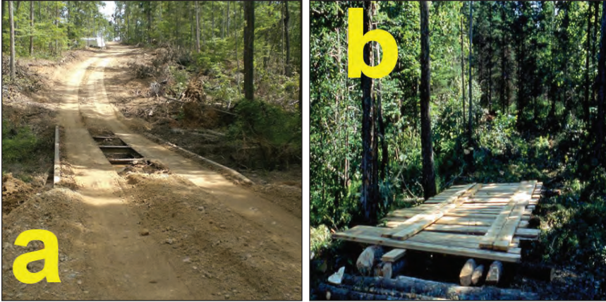
Figure 8.7. Aluminum truck bed modified for crossing use (a), and pole and lumber skidder bridge (b).
