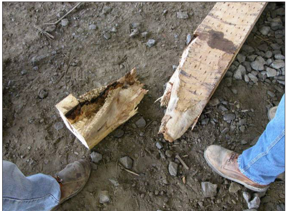
Figure 14. This tie broke when I picked it up. There was a combination of slope of grain and decay here.
